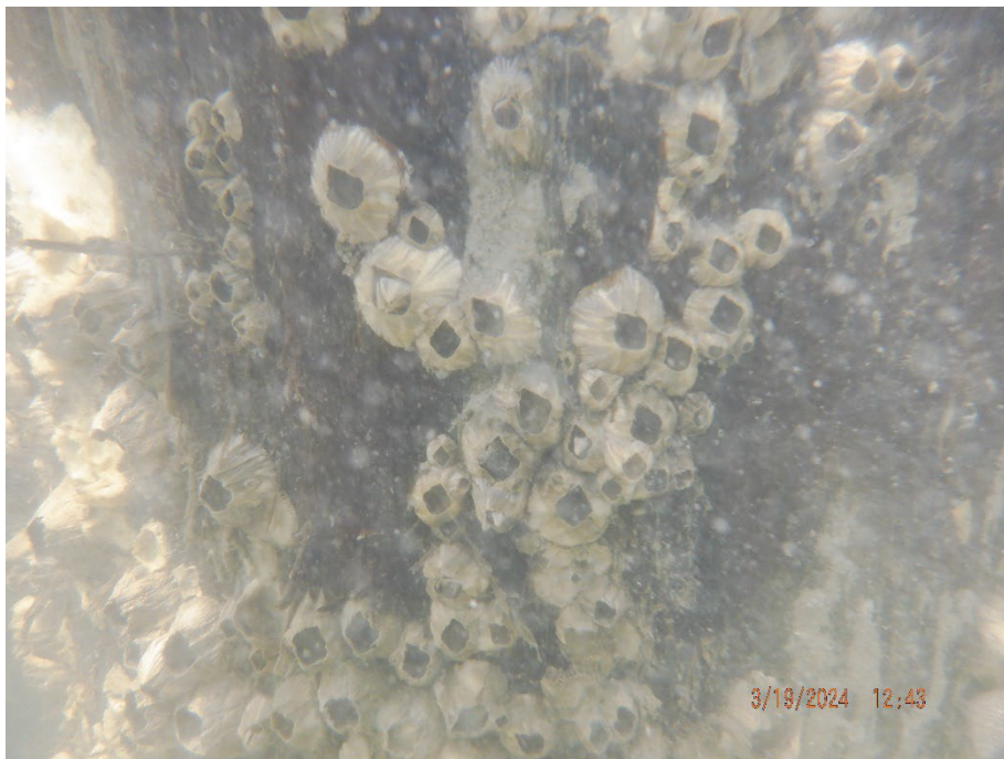
Figure 2: View of barnacles observed on the existing pilings.
